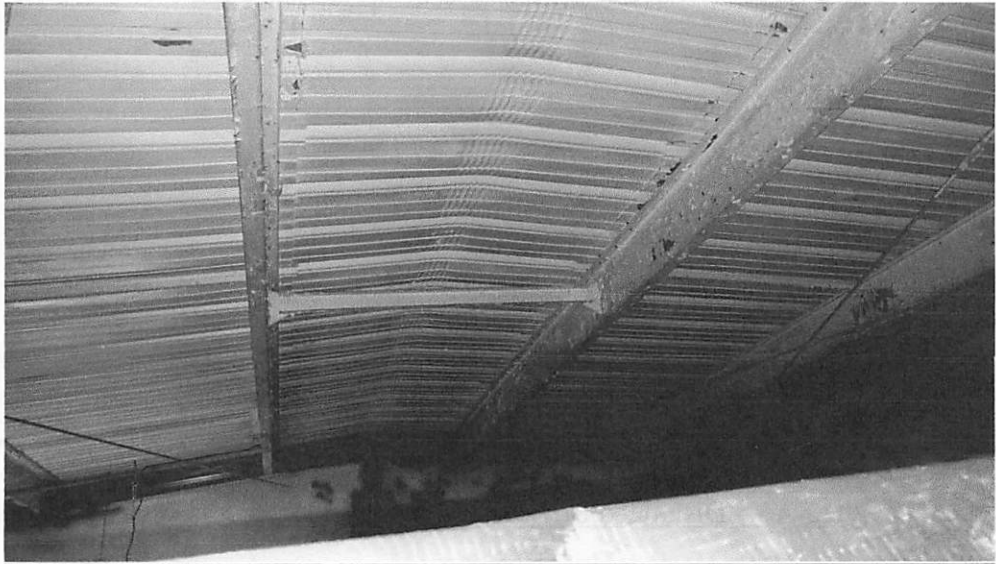
2022-A4 – Paint peeling from Roof Purlins and Main Girder
