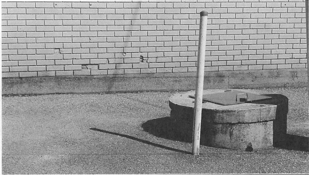
2022-A5 – Damaged Brick on Front Elevation
